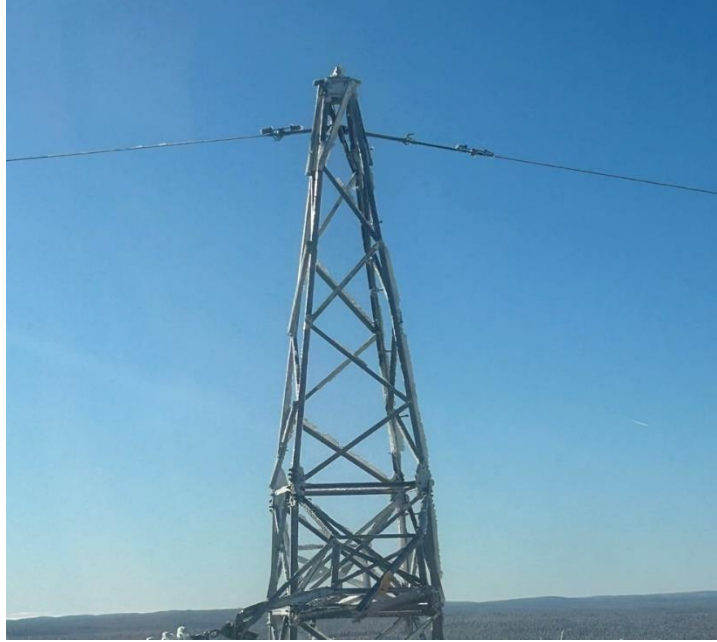
Figure 7: Pulled OPGW due to Ice Removal
