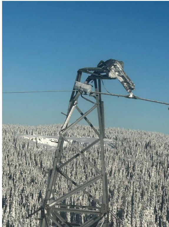
Figure 6: S120/121 OPGW Peak Failure due to Ice Removal
