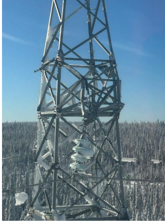
Figure 5: S130 EL1 Cross Arm Failure
