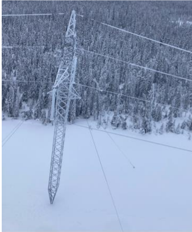
Figure 10: Ice conditions at Time of Helicopter Patrol Discovering Damage
