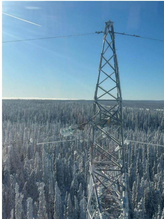
Figure 4: S128 EL1 Cross Arm Failure
